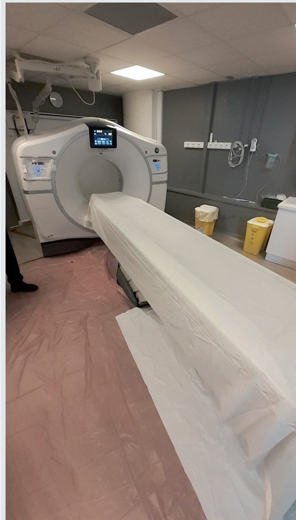
Figure 3: CT Scanner and floor of the CT room covered with vinyl sheets
